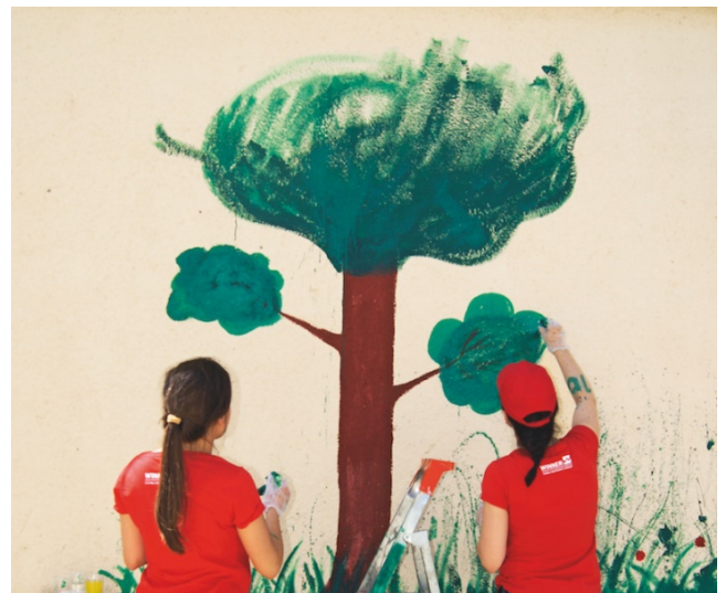
Winner Non-Life and Life employees renovated the outdoor facilities of an SOS Children's Village in Macedonia on their Social Active Day © Winner
